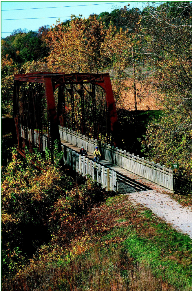
Bridges like this on the Katy Trail are in need of repair.
